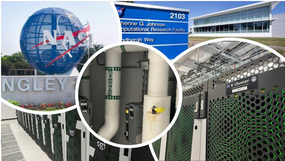
Figure 5: Langley’s High-End Compute Infrastructure (as of August 2023)
